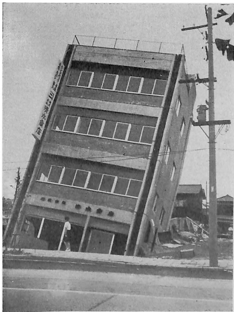
Fig. 5. Tilting of a multistoreyed building due to liquefaction of soil during Niigata earthquake (1964) in Japan.
