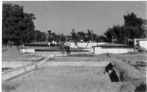
Institutional Type Biogas plant.
