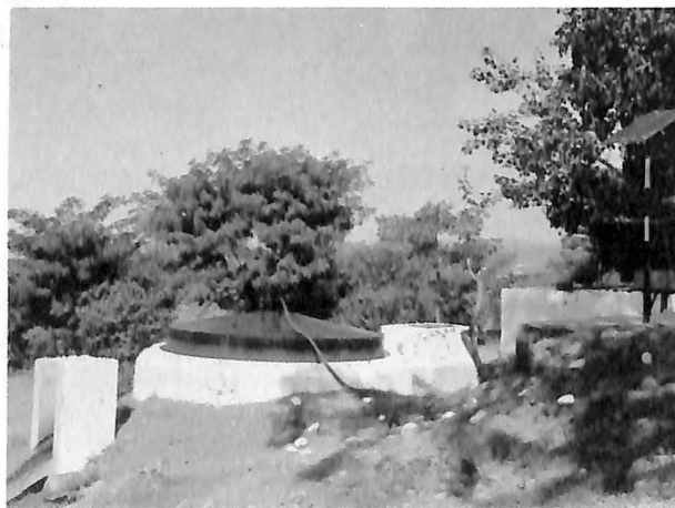
Community Type Biogas plant in a village, Jammu and Kashmir.
