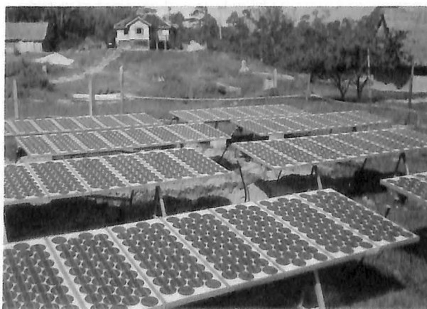
A 5 kW SPV power plant installed in Andaman & Nicobar Islands.
