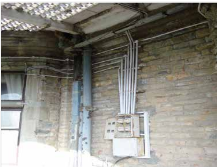
Structural damage of Oriel windows due to leakage and seepage from prism glass ceiling and new interventions
