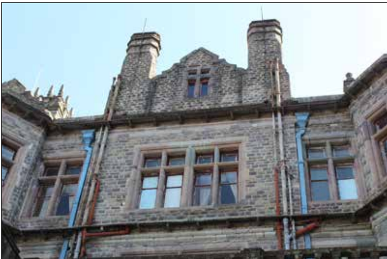
Exterior view from the north showing top two floor levels with chimney stacks
