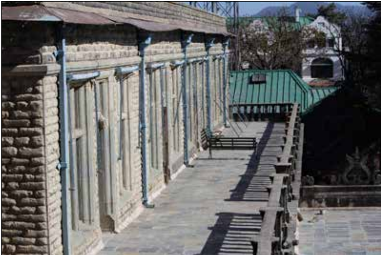
Removal of dead and decayed mortar on the joints of the stone tiles paving on flat roof for repointing
