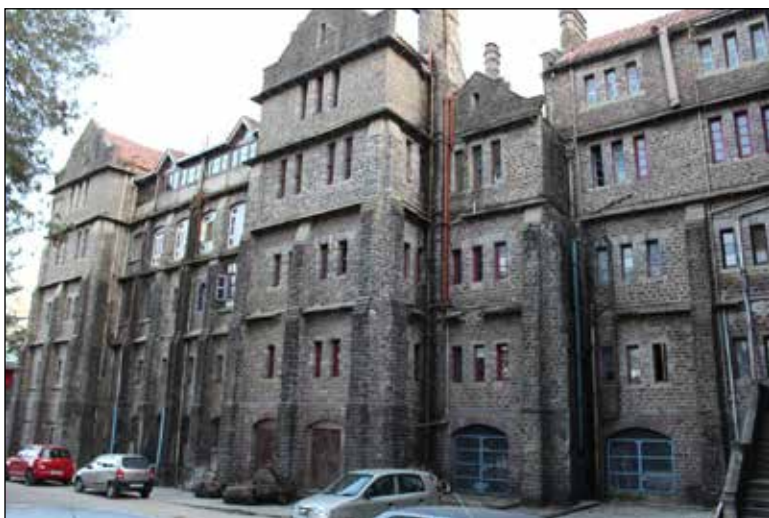
Exterior north view of the Kitchen Wing showing damaged downpipes and chhajas, etc.
