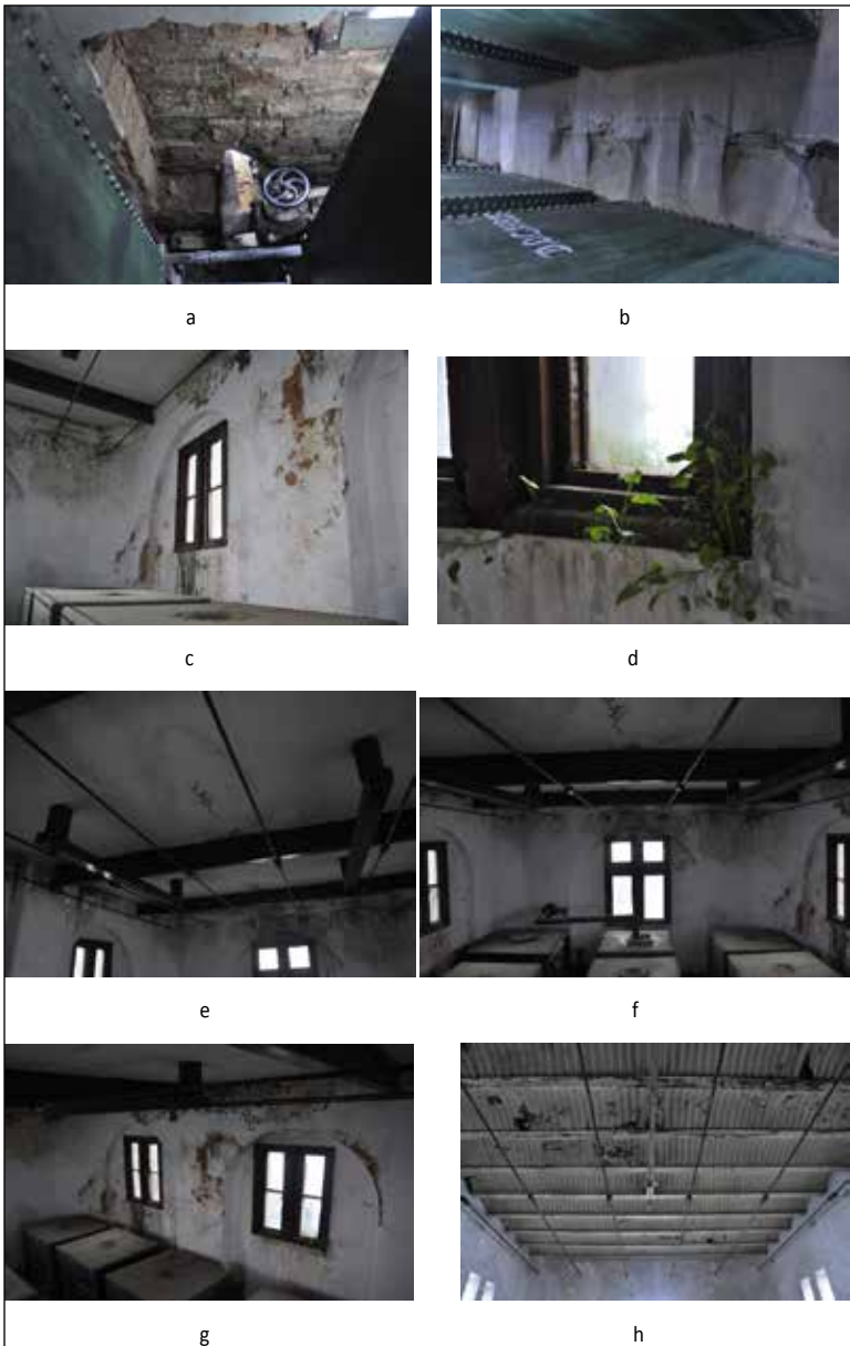
Interior distressed conditions of the Central Tower.
