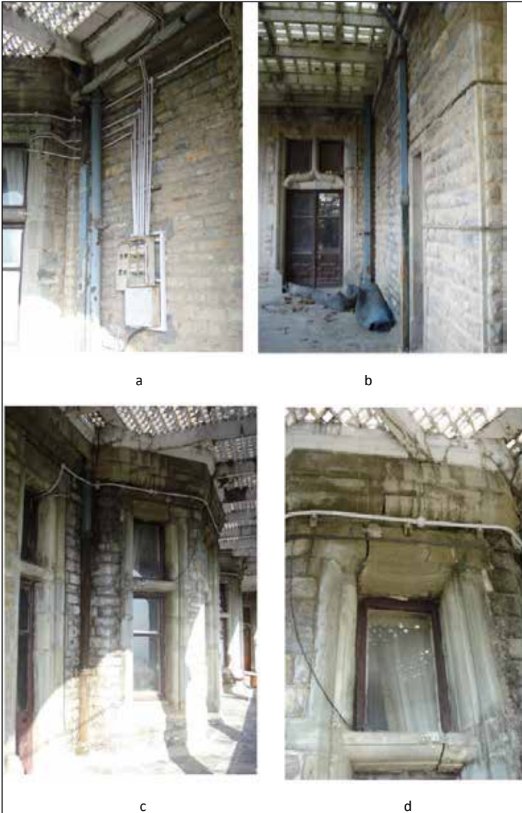
Structural damage due to water penetration from broken and missing Hayward Glass ceilings
